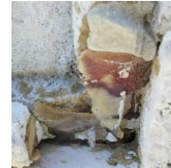
(A) Resin Repair (incompatible)
