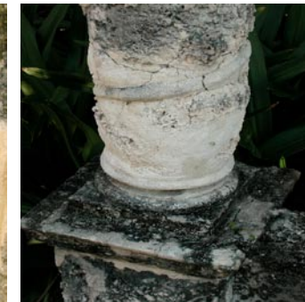
(B) Mortar Repair (left - incompatible) (right - compatible)
